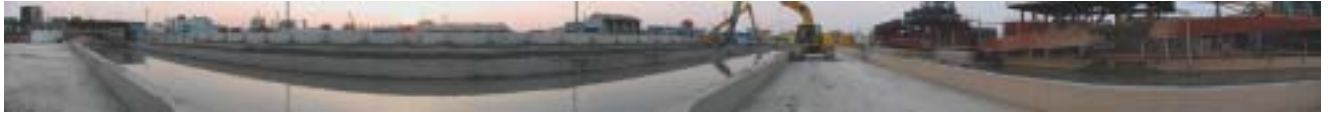
Tunnel construction site in Shanghai with sludge sediment reservoirs and pumping station
