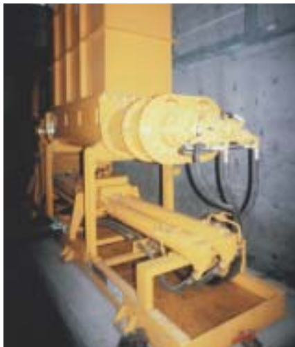
KOS 1470 HP with THS 842 HCB pumps the sludge from the drainage point to the silo
