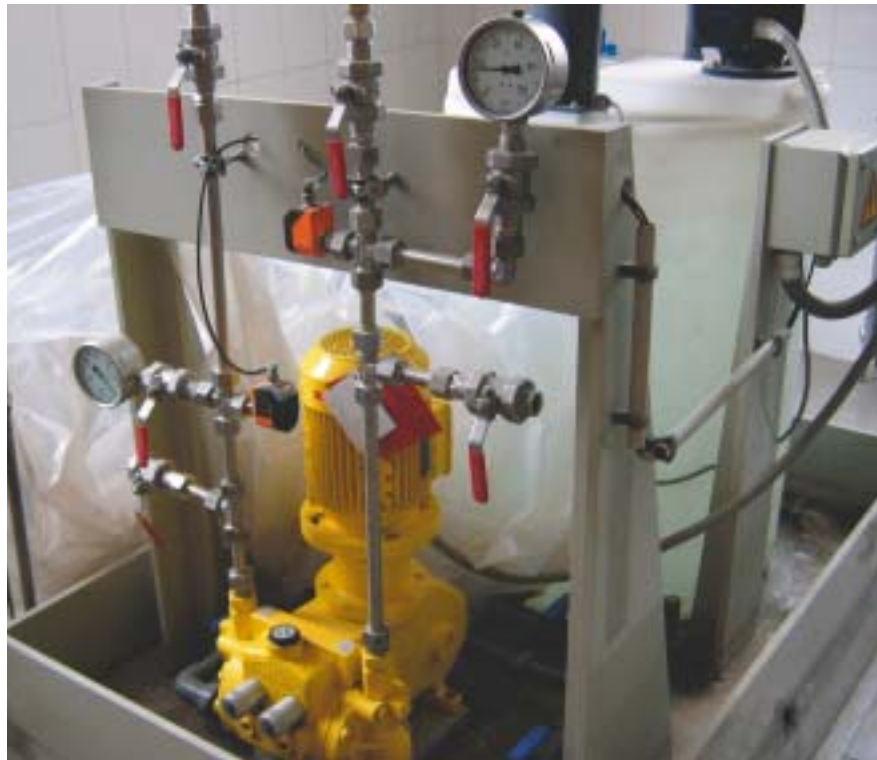
BLI dosing station with mixing tank and control equipment
