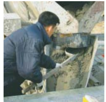
The mixer driver has to really scrape the remainder of the relatively stiff concrete off the chute
