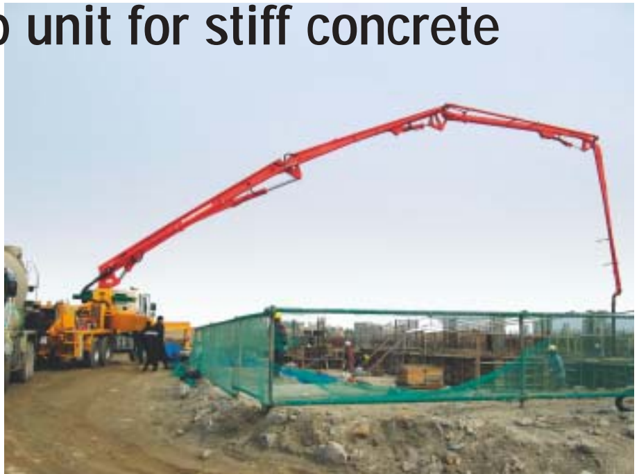
A lot of work to be done at the goods terminal of Gimpo Airport: the Putzmeister BSF 36.16 H, produced in Korea
