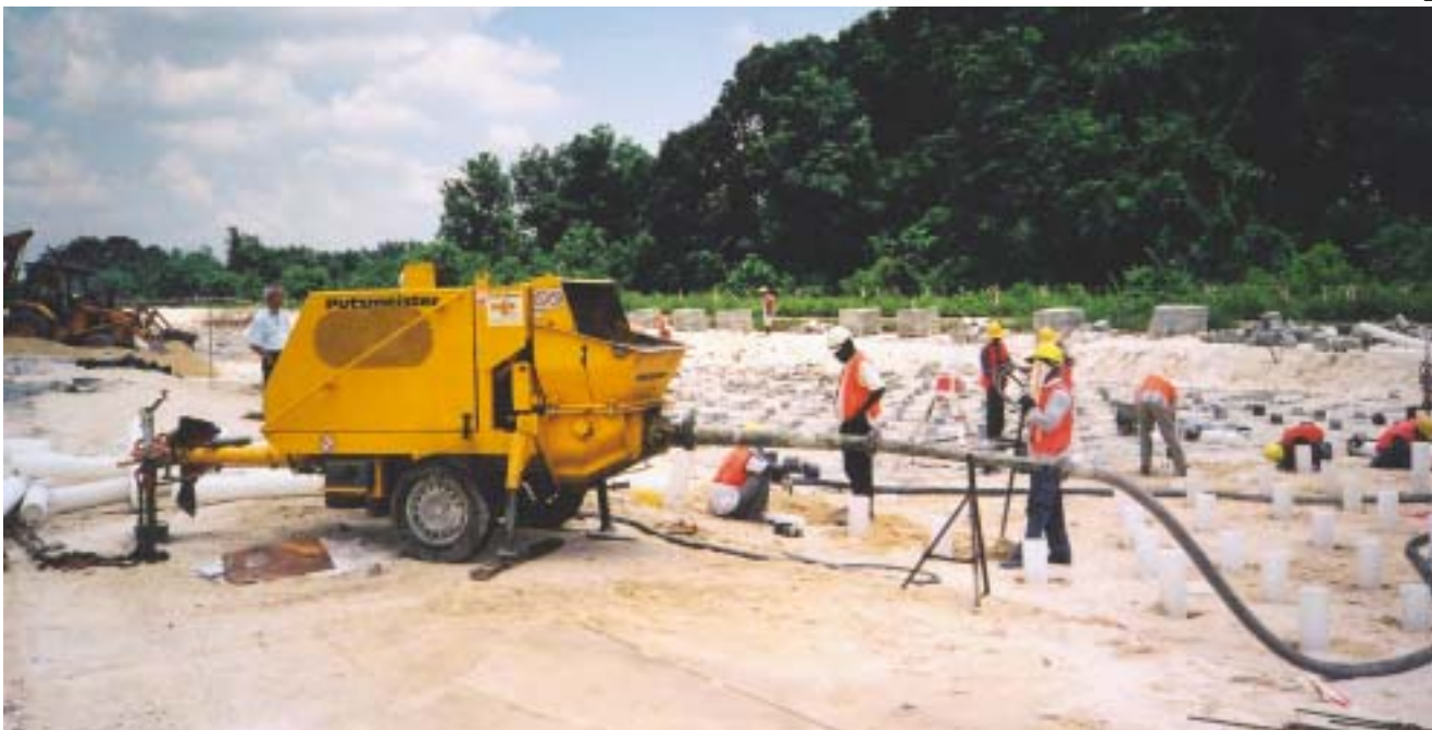
The Putzmeister trailer concrete pump BSA 1002 D conveys the cement mortar via a reduction pipe and flexible hoses into the plastic pipes which had been previously pressed into the ground
