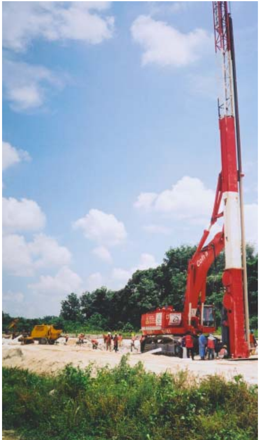
A special gun presses the plastic pipe which is protected by a steel casing, into a depth of 25 m
